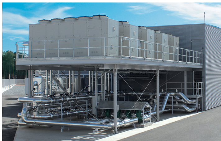
T-Systems' Prefabricated Modular Data Center in Spain
